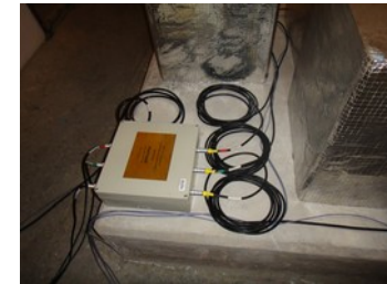
Metrozet E300 electronics box
